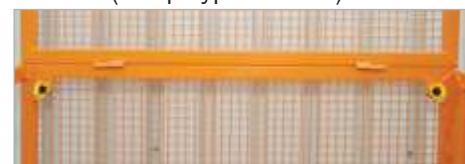
anchorage points for protective equipment
